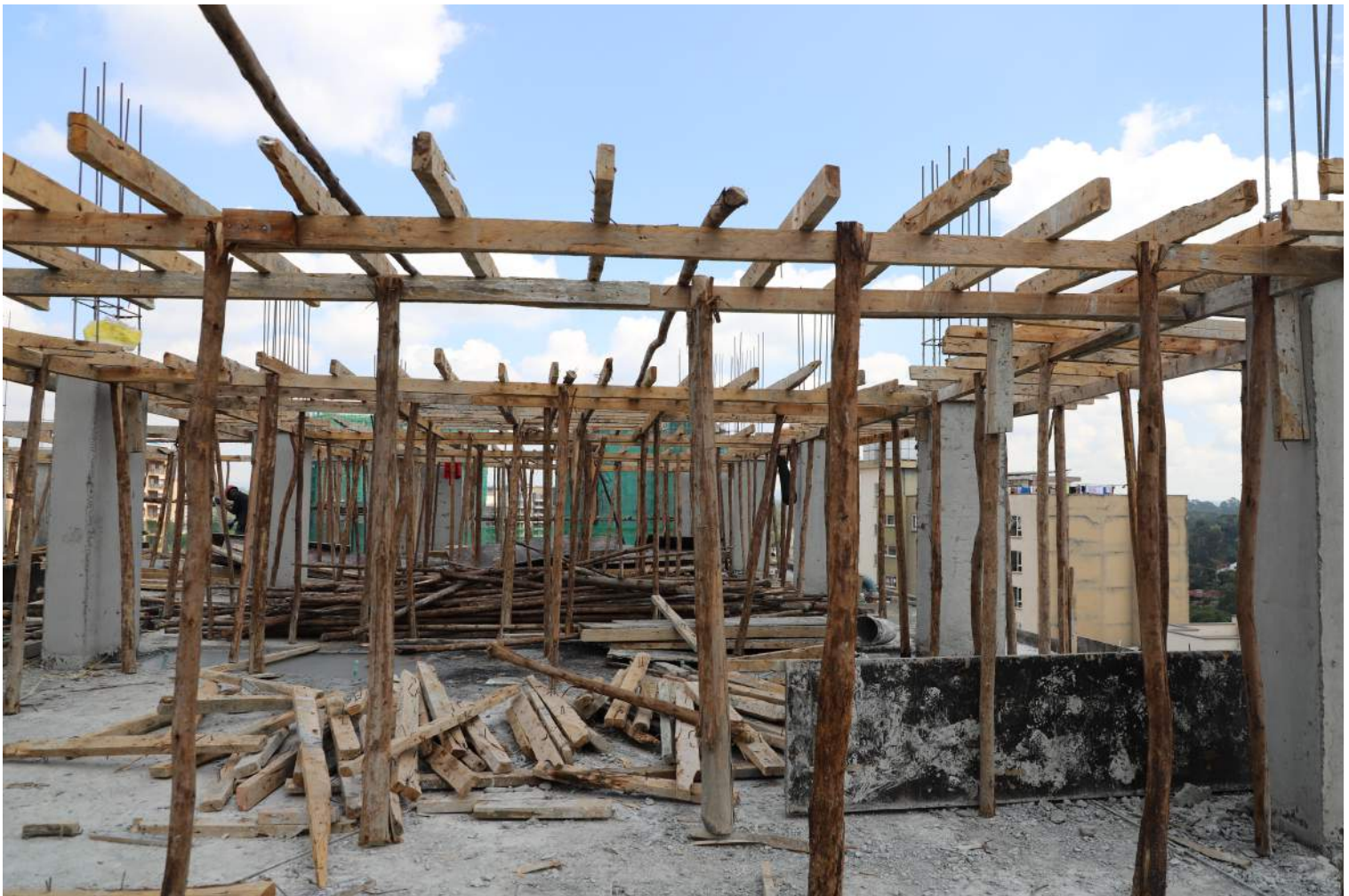
Shattering of the 13th floor and column bases
